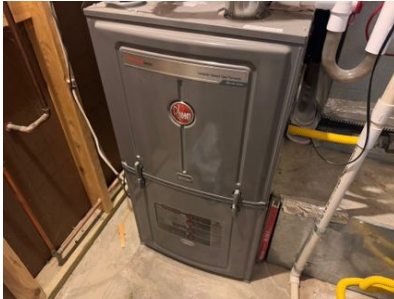
Gas furnace exterior
