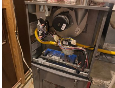
Gas furnace interior
