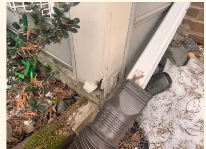
Wood rot close to the downspout
