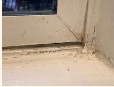
Sealed shut with caulking
