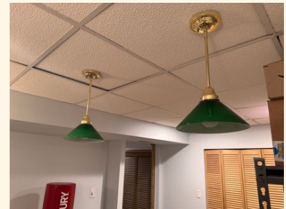
Basement light fixture
