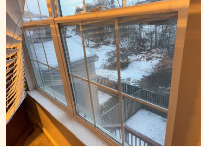
Main bedroom windows do not stay open
