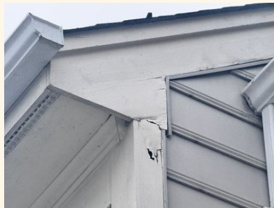
Wood decay in fascia material
