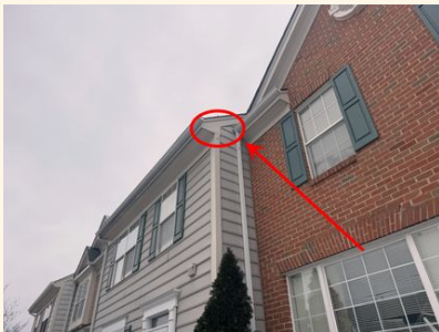
Wood decay in fascia material
